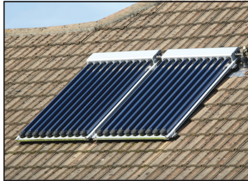
Solar water heater
