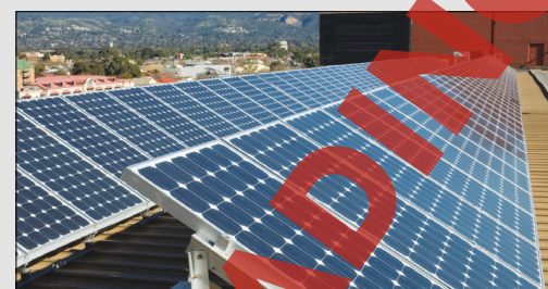
These are called solar cells. The Sun beats down on them. They take in energy from the Sun. They change this into electricity.
